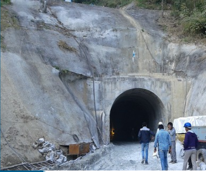
3 x 4 MW Hydro Electric Power Plant— 1, East India (Above & Right)
